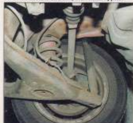
At the rear, check out the driveshaft gaiters, mounting bushes for the rear sub-frame/trailing arms, and condition of the steel suspension components. Deficiencies here spell MoT failure.
